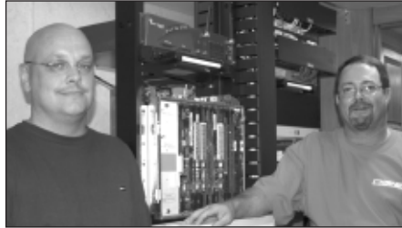
Steve Redgewell (l), support manager, Prizm USA, and Bob Funk, sales engineer, Tadiran Telecom, Inc., discuss the new Tadiran system that GCC installed at Prizm USA.
